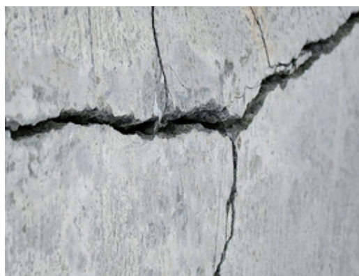
© stone crack, Fotolia #3669926
